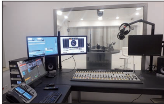
Digital IP Radio Control Room
