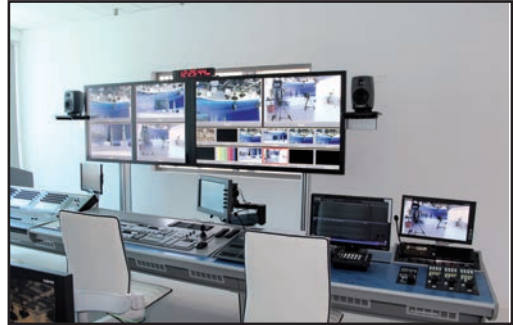
HD TV Studio Control room
